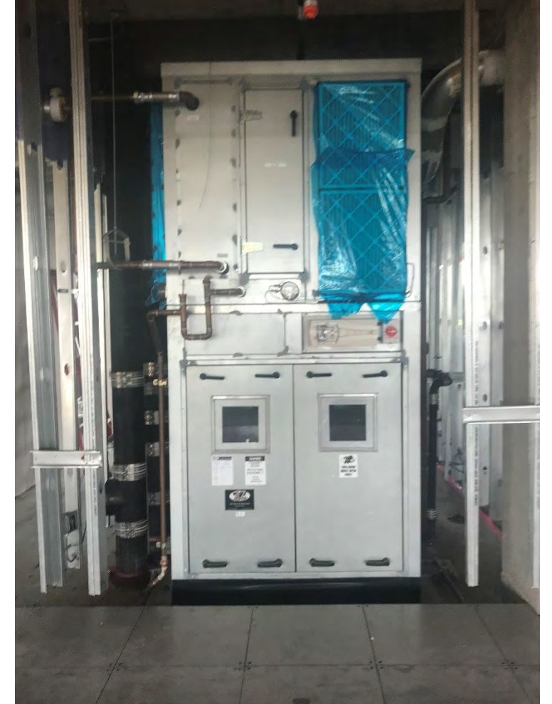
Typical Air Tower (One of Three Per Floor)
