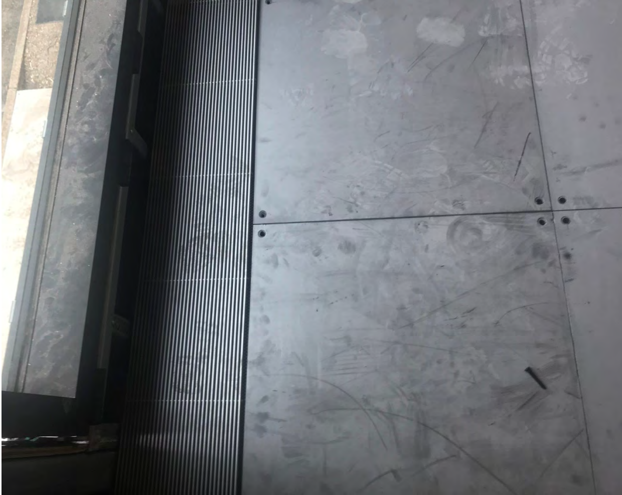
Perimeter Fan-Powered Boxes
